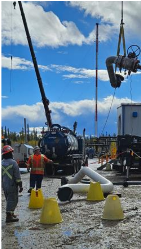
Demonstrating: Tag line use, spotter/communication with crane/clear line of sight with operator/rigging.
